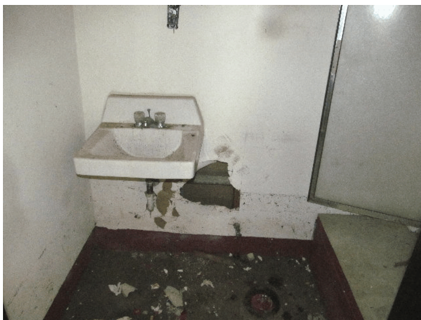
12. Restroom in front store/office area, again illustrating the building's dilapidated condition.
