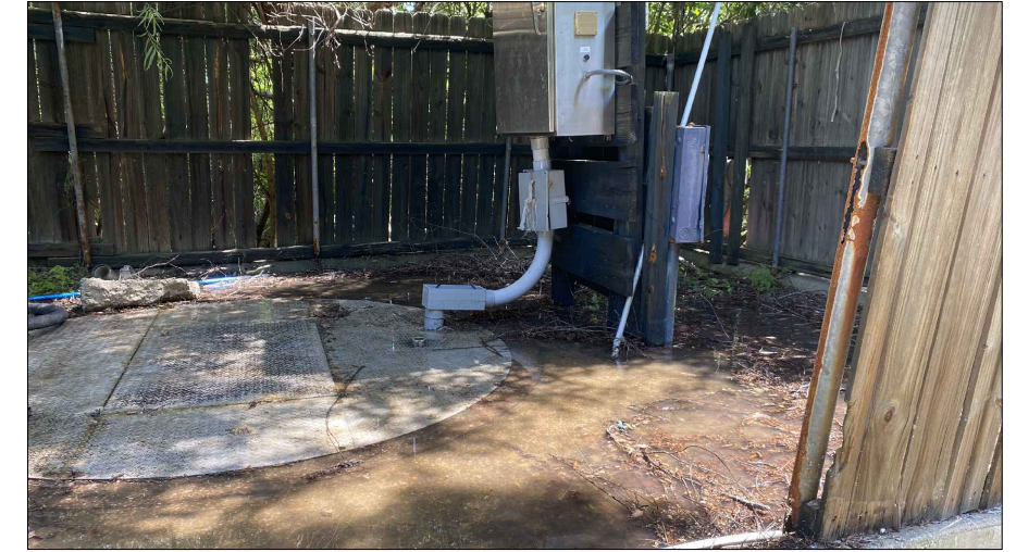
Wet Well Overflow
