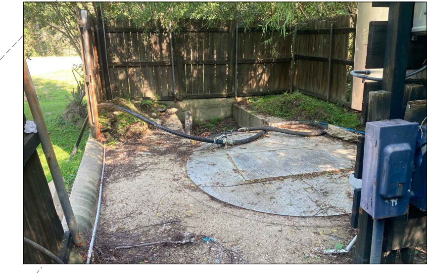
Wet Well - Looking West
